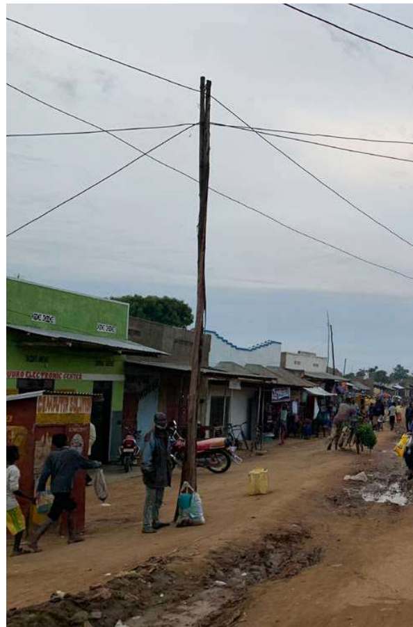
Fig.51: Informal Electricity Network in Base Camp
