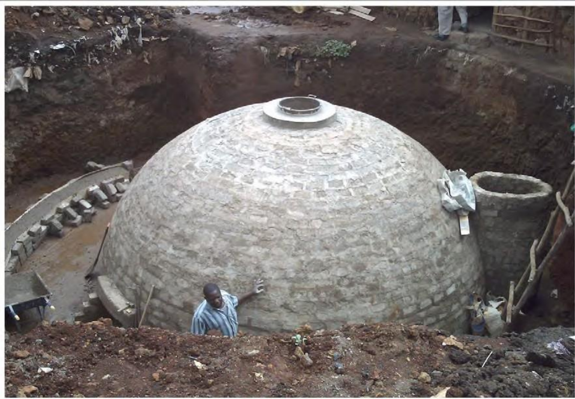
Biogas Digester under construction by Umunde Trust, in Nairobi. A Bio center is constructed over the digester with public toilets on the ground floor and a kitchen, office and meeting room on the first floor. Power and cooking fuel are derived directly from the gases generated from the urine and feces derived from use of the public toilets and stored in the dome.
