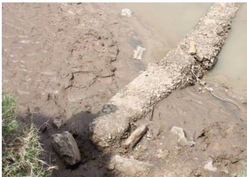
Photo 33: A sub-surface dam that cracked due to subsidence
