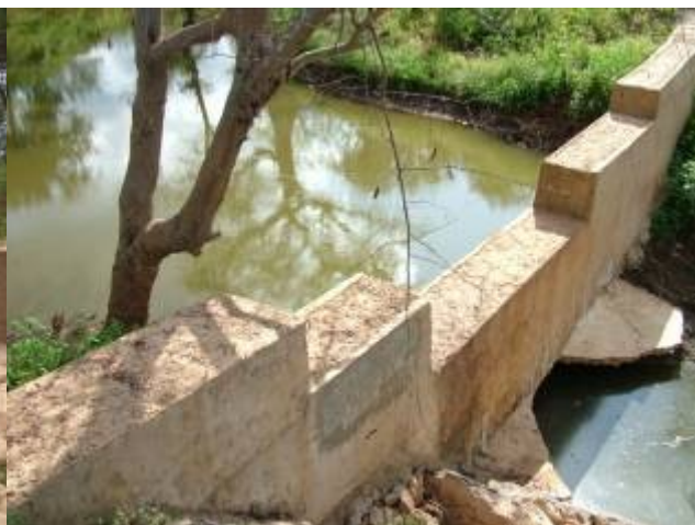
Photo 40: Sections of the apron have been undermined due to foundation and size of the apron being inadequate.
