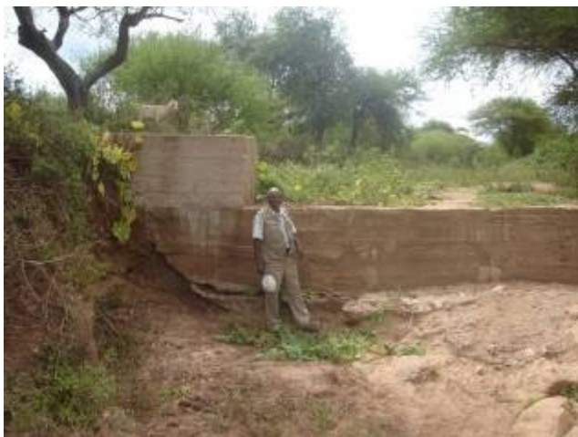
Photo 39: Erosion of left hand bank shows the foundation and apron do not extend into the riverbanks
