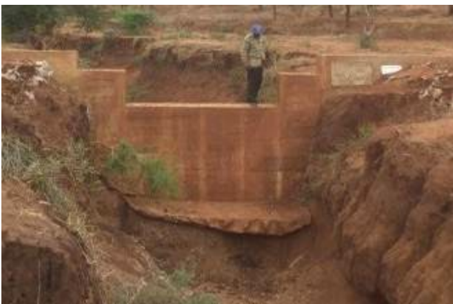
Photo 37: Examples of poorly constructed dam aprons
