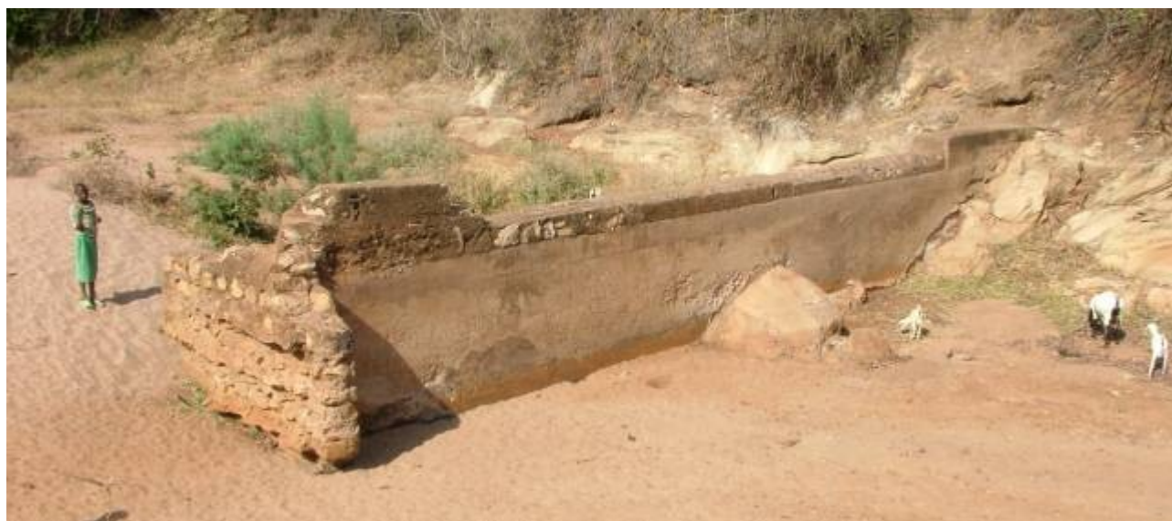
Photo 16: A failed dam near Mtito Andei, Kenya
