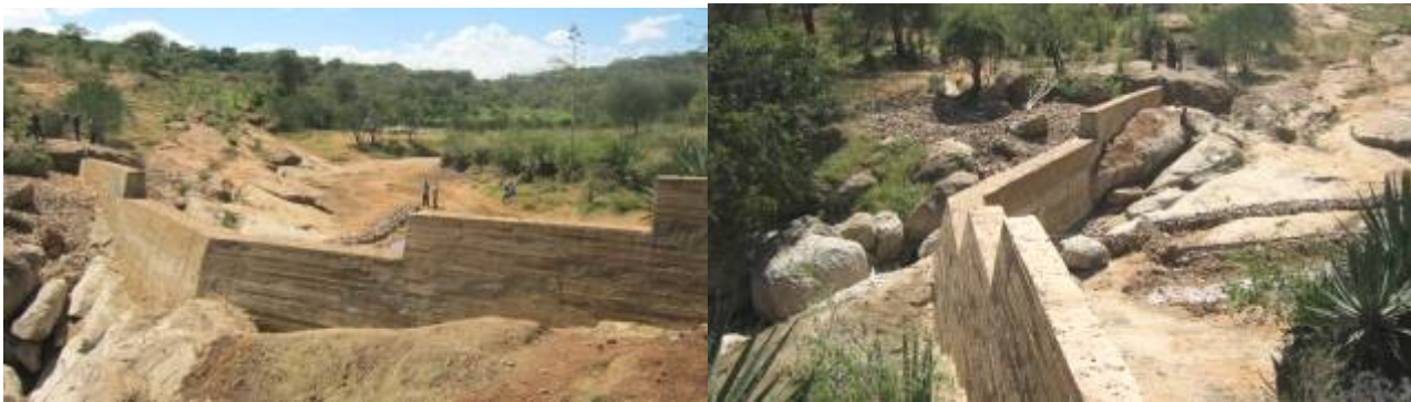
Photo 19: Dam angled to follow the bedrock and bring the flow back to the centre of the river
