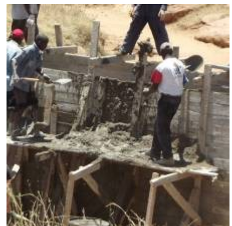
Photo 36: A raised platform allows the mortar to be thrown into the formwork
