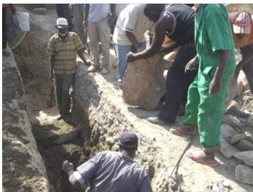
Photo 35: Where the dam sits in a trench, the trench walls are used as formwork (NB flip flops)
