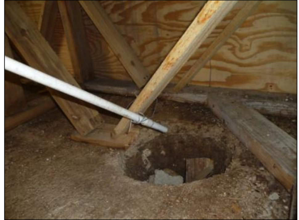
PHOTO BAD T6: Poorly installed drainpipe not entering into soakaway pit.
