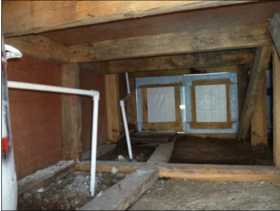
PHOTO BAD T5: Early plumbing with 90 degree bends causing drainpipe blockages.
