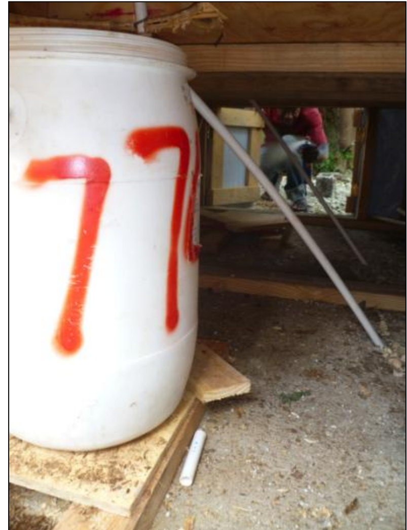
PHOTO T2: Drum in position beneath poophole
